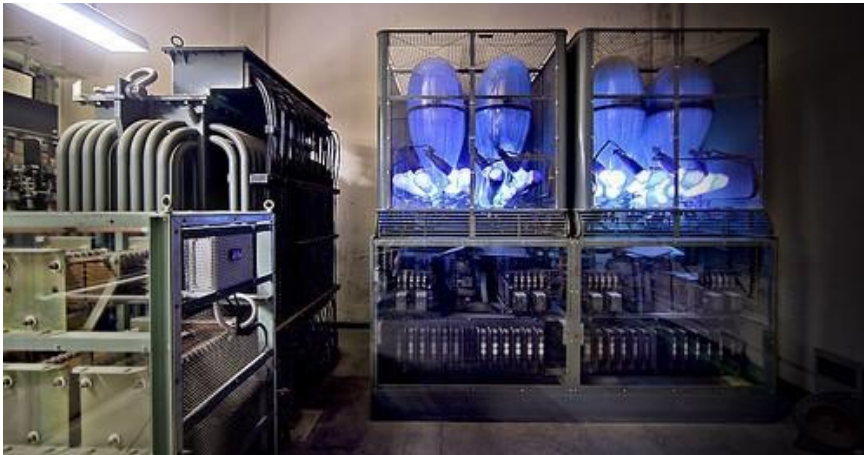
Mercury Arc rectifiers in Russell Place substation formerly produced direct current for trams from the AC transformer at left.
