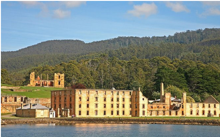
Port Arthur convict settlement Tasmania. Under-fired brick subject to salt attack causing deterioration.
